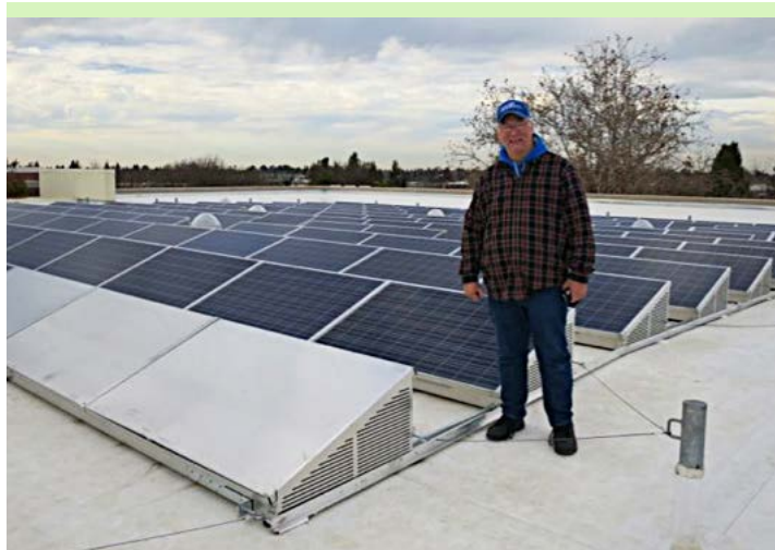
Rick Stewart stands next to the solar panels atop the Winn Center.
